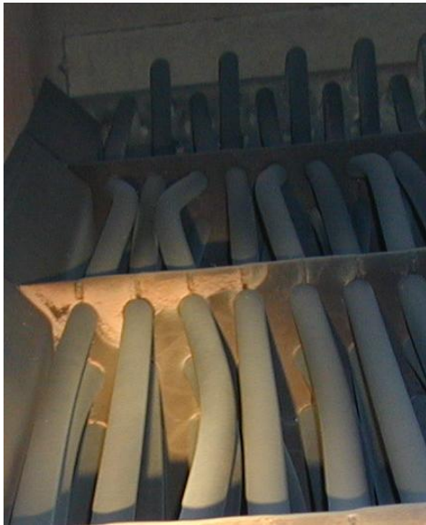
Deformation of economizer tubes
